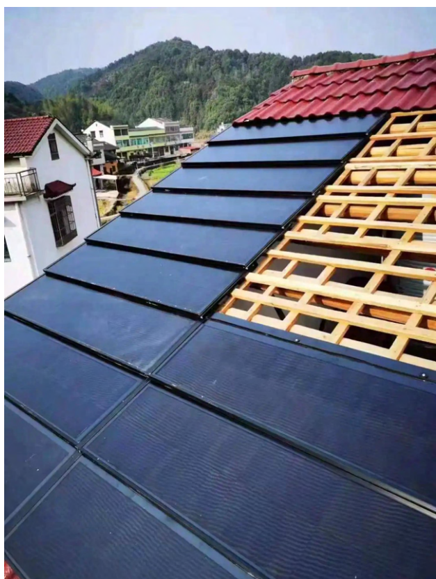
An example of an on-going installation of Flat solar tiles on a house roof.
